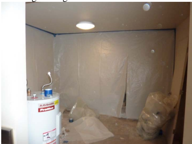
Prepping for renovation of new bathroom and flooring in Stewart House apartment
