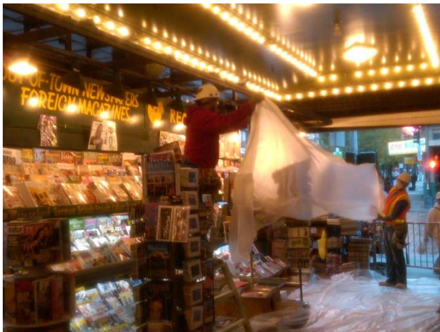
Emergency Lighting Revisions
