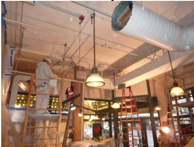
Duct work in De Laurenti's
