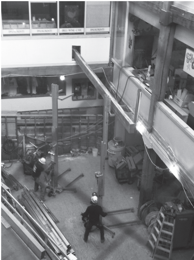
Left: Installing a 22 foot drag strut (used to connect the walls of the building) inside DeLaurenti's.
