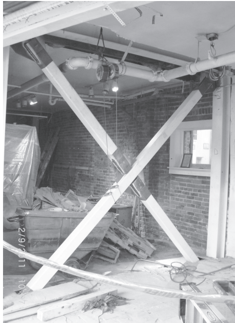
An example of the steel seismic bracing. This brace frame will be hidden in the wall between Mr. D's and La Buona Tavola in the Triangle Building.
