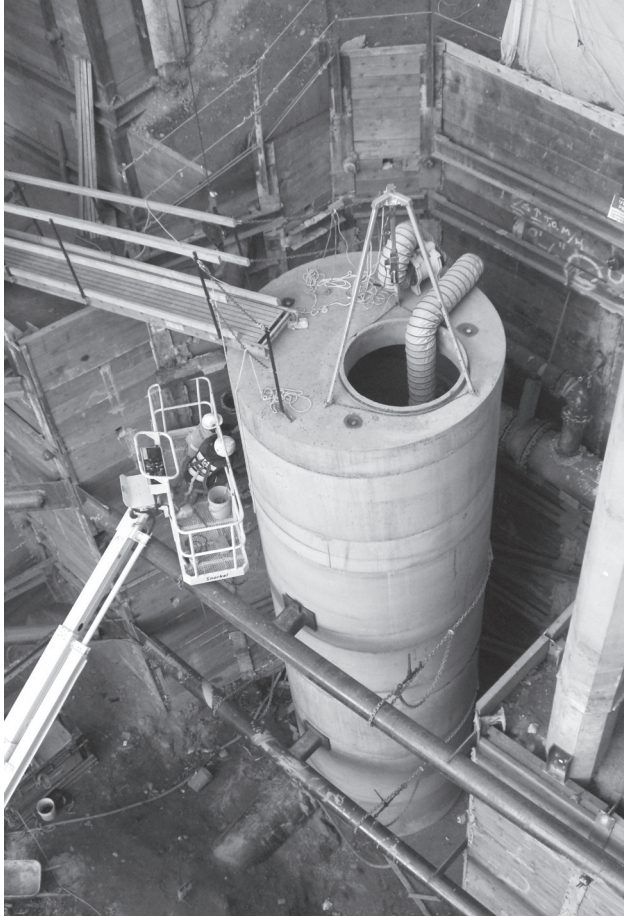
This new sewer manhole, located on the Market Hillclimb off Western Avenue, is 10 feet across and 43 feet tall. It houses sewer lines from the Market as well as the sewer main from First Ave. John Turnbull noticed that in this picture, the manhole resembles the world's largest soda can!
