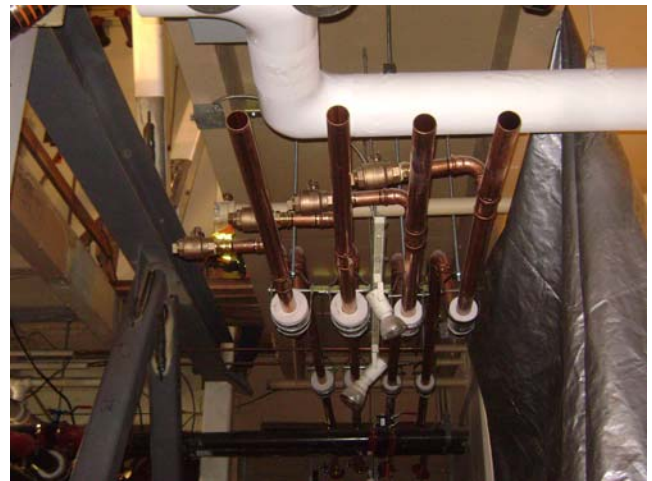
Piping in the Sanitary Market
