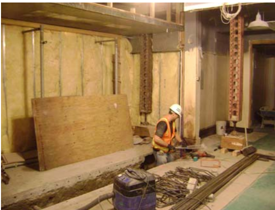
Ready to begin Ice Box footing for the Brace Frame installation in Kitchen Basics
