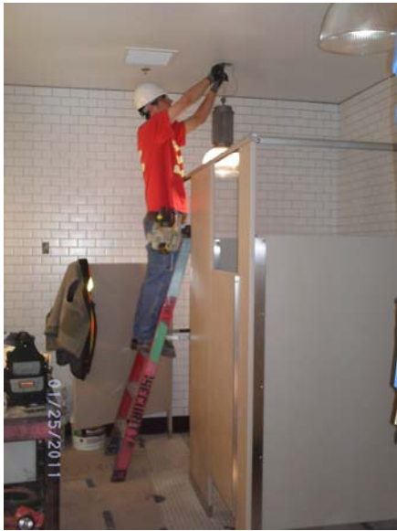
Lighting in Women's Public Restrooms-Sanitary Building
